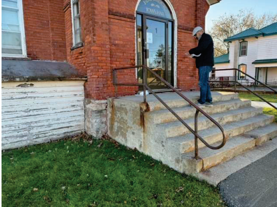
Photo #71 Town Hall Entrance Concrete Stairs. The concrete exhibit signs of spalling, potential water damage, and corrosion on the handrails.
