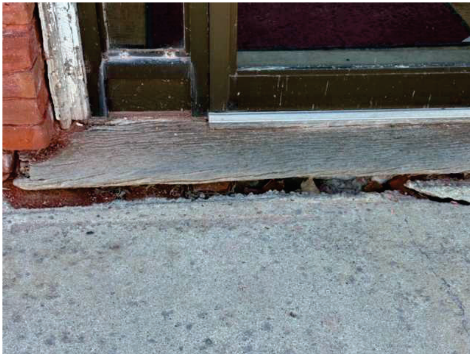
Photo #72 Entrance door threshold exhibits signs of settlement, with visible gaps and crumbling materials. The wooden threshold is weathered and misaligned.
